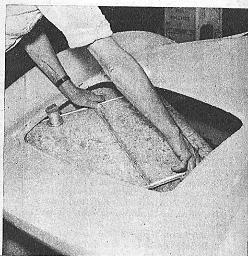
3.—Fuel tank, under boot, will be covered by flat floor. Outlet and gauge unit are positioned to match existing connections.
